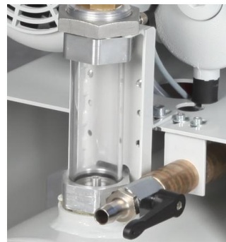
Sight glass (Liquid level)
